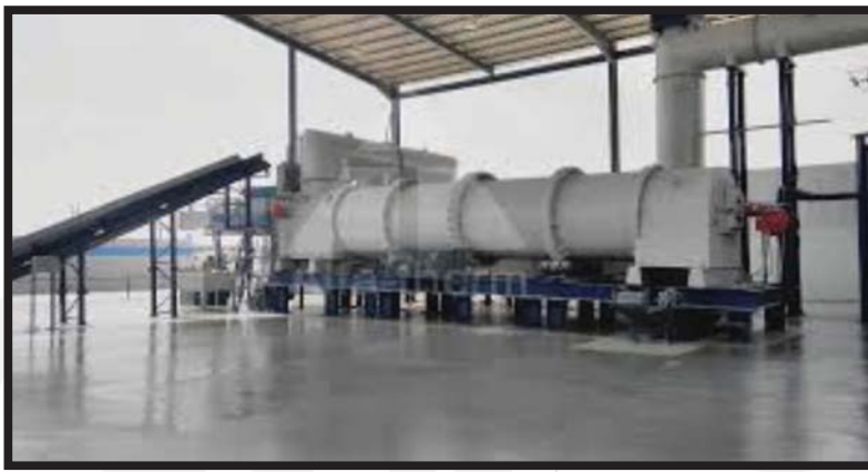
Fig. 20.3: Rotary Kiln Incinerator
